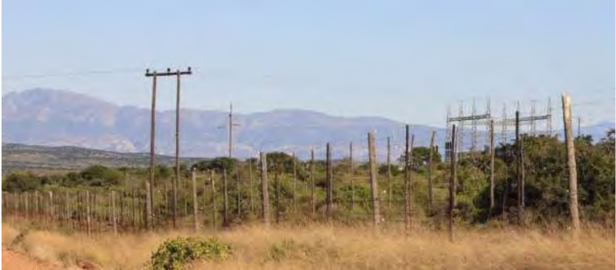
Figure Error! No text of specified style in document. -29 Small substation with overhead power lines and pylons against the mountain backdrop (RVP011).
