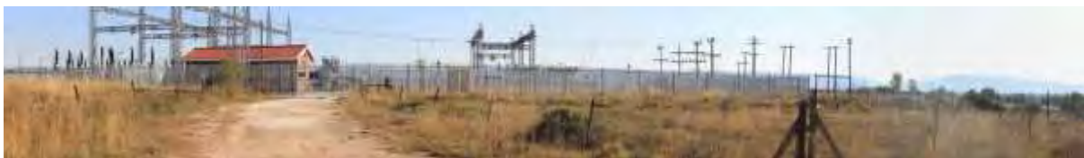
Figure Error! No text of specified style in document.-36 Substation next to the R75 where the proposed 132 kV line will connect with the Eskom grid.
