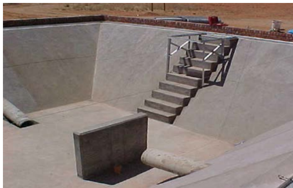
Plate 5 Oil holding bund
