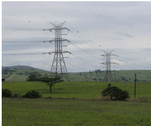
Plate 6 Double-circuit 400 kV transmission line
