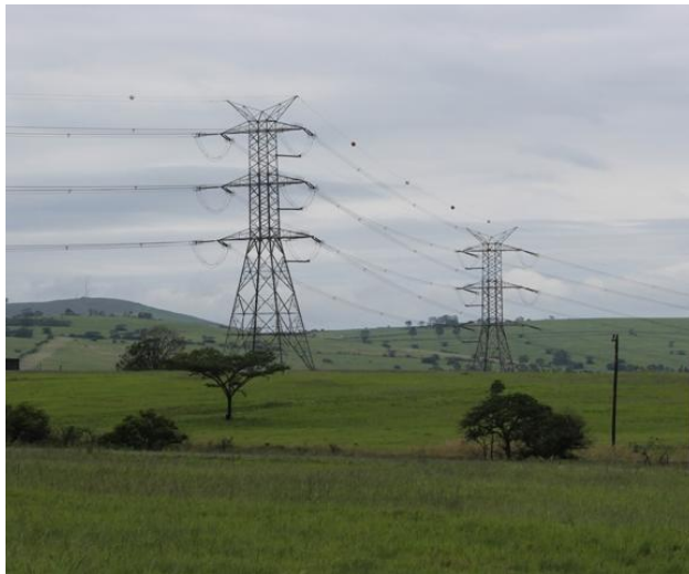
Plate 6 Double-circuit 400 kV transmission line
