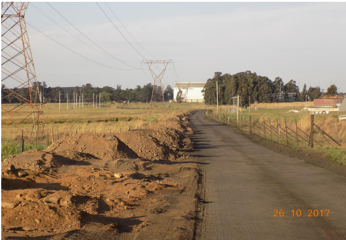
Figure 2: View of the condition of the existing road
