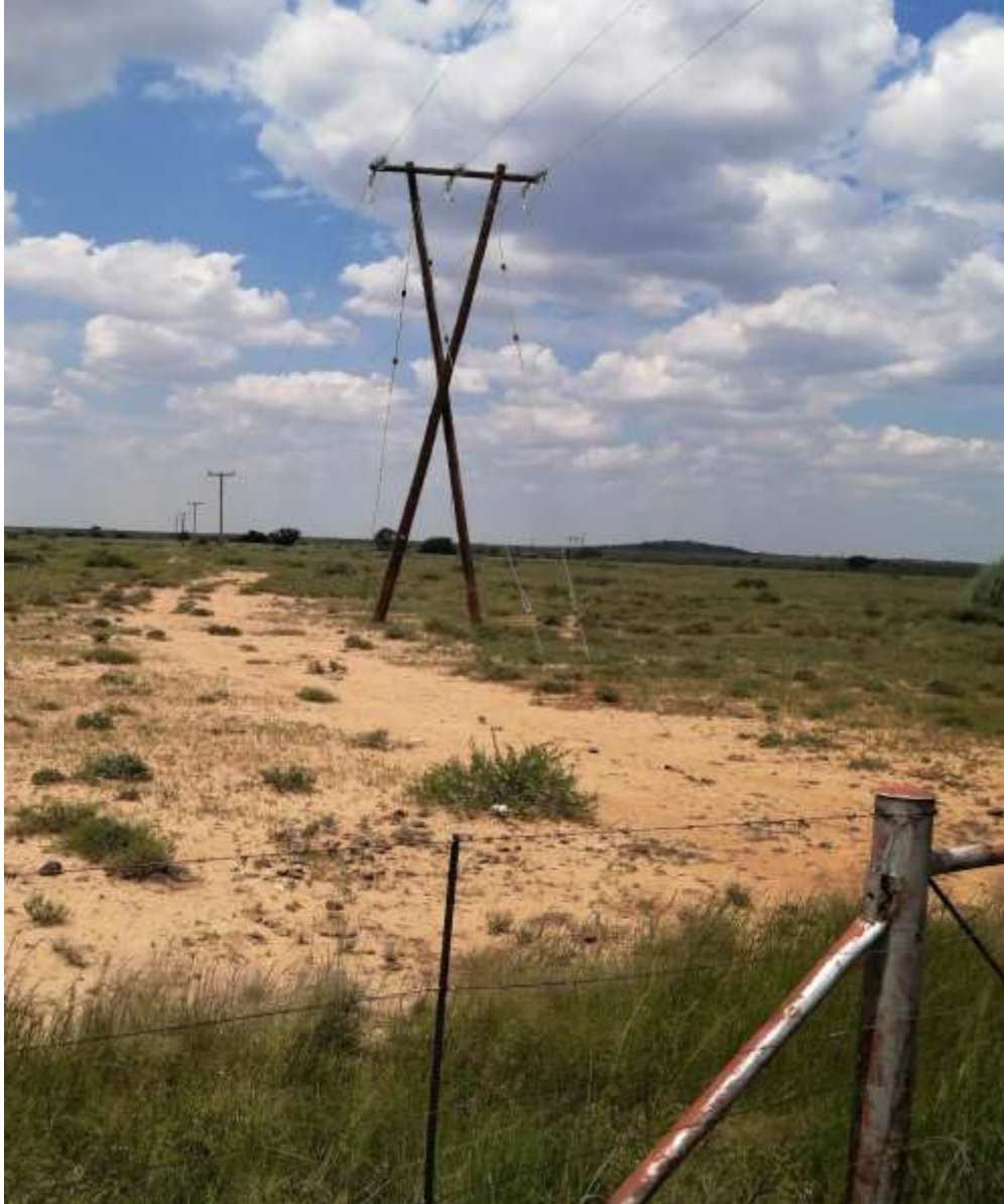
Figure 14: Existing 22kV power line at line termination
