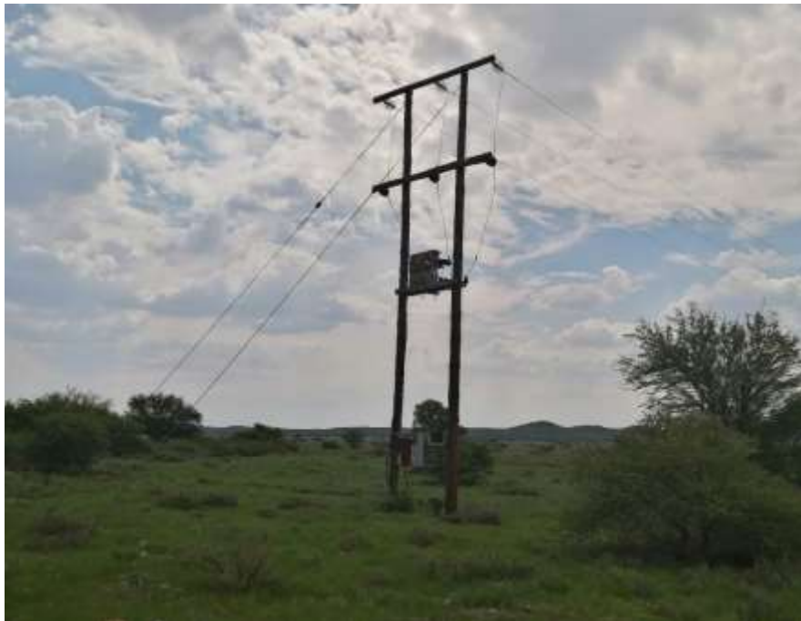
Figure 14: Existing transformer pole
