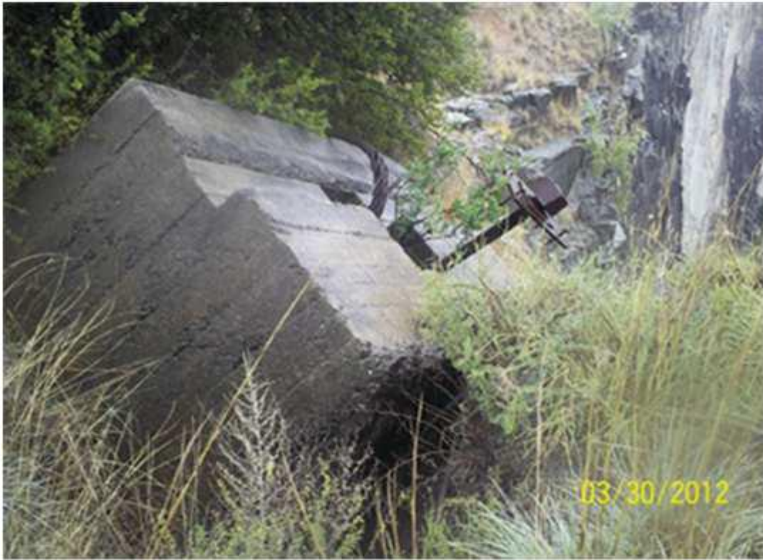
Figure 5: Old undermined installations.
