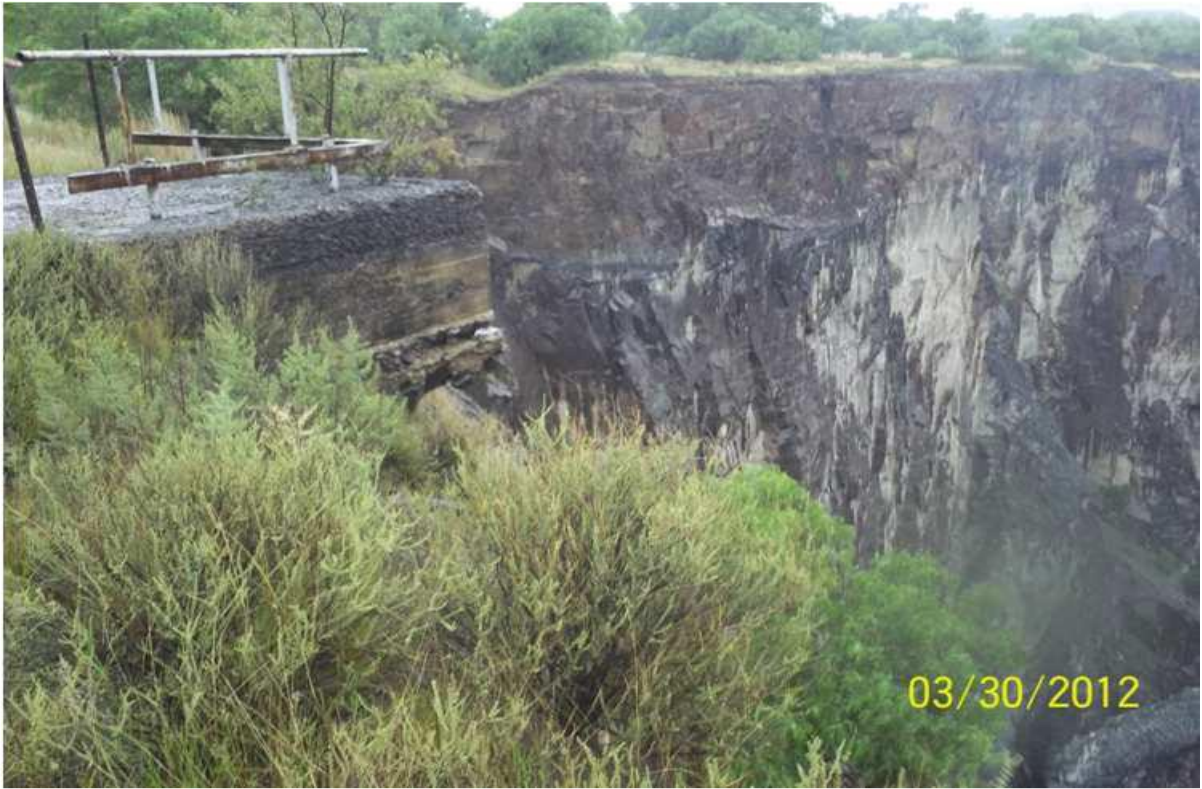
Figure 4: Condition of the outlook position.
