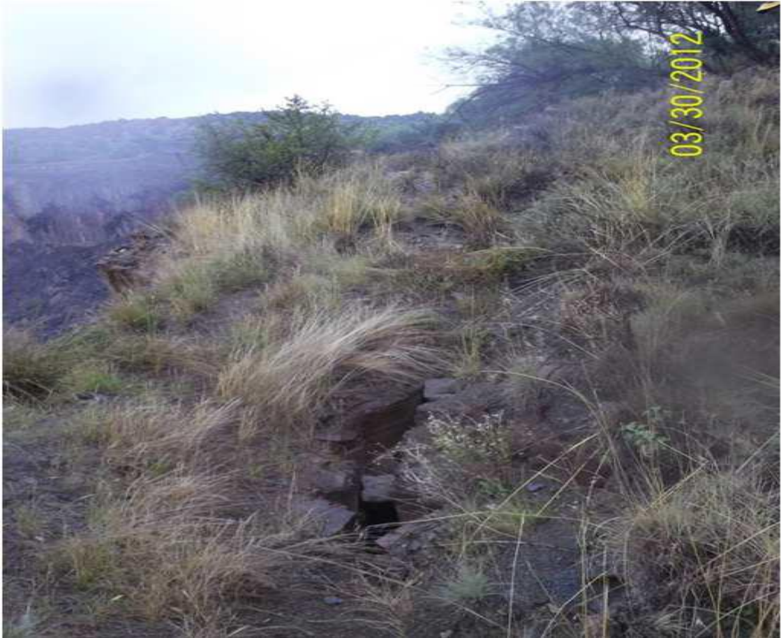
Figure 7: Numerous cracks at distance of 5m 10m from the edge of open Pit.
