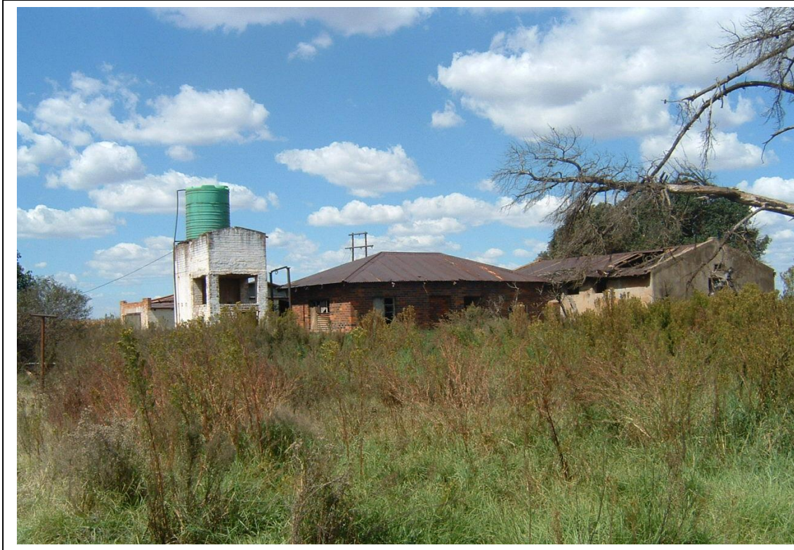
Figure 18 A water stand, house and shed on Wolwenfontein 488. These structures, particularly the residence, are in a severe dilapidated state and has become structurally unsafe.
