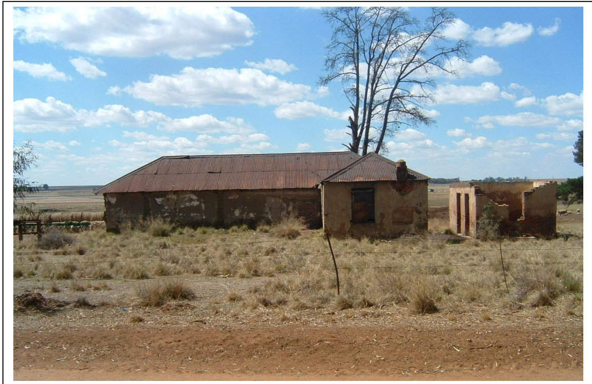
Figure 16 Site no. 15 consists of a historical house outbuilding on Wolvenfontein 244. These structures are severely dilapidated.
