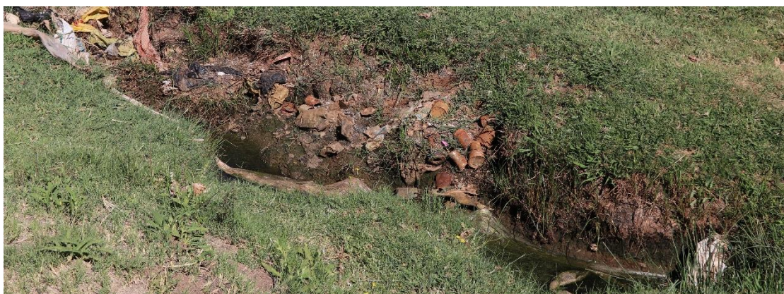
Figure 30: Close-up of the main channel illustrating a high amount of refuse, algae concentrations and an odour which indicates the presence of raw sewage.
