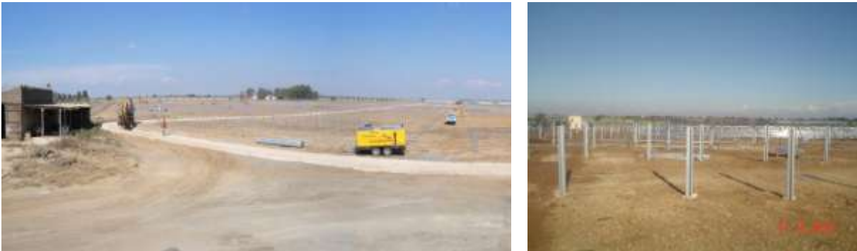
Figure 31: Showing typical examples of site preparation during the construction phase of the project (Solek, 2013).
