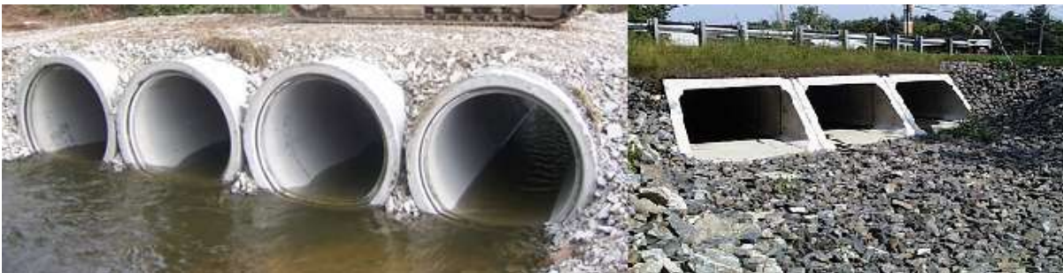
Figure 38: Showing examples of temporary measures for the potential crossing of the main drainage channel on site (Solek, 2013).
