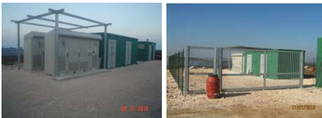
Figure 28: Typical example of on-site substation and transformer (Solek, 2013)
