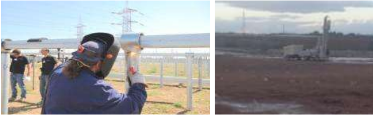
Figure 32: Showing typical erection of PV panels during the construction phase of the project (Solek, 2013).
