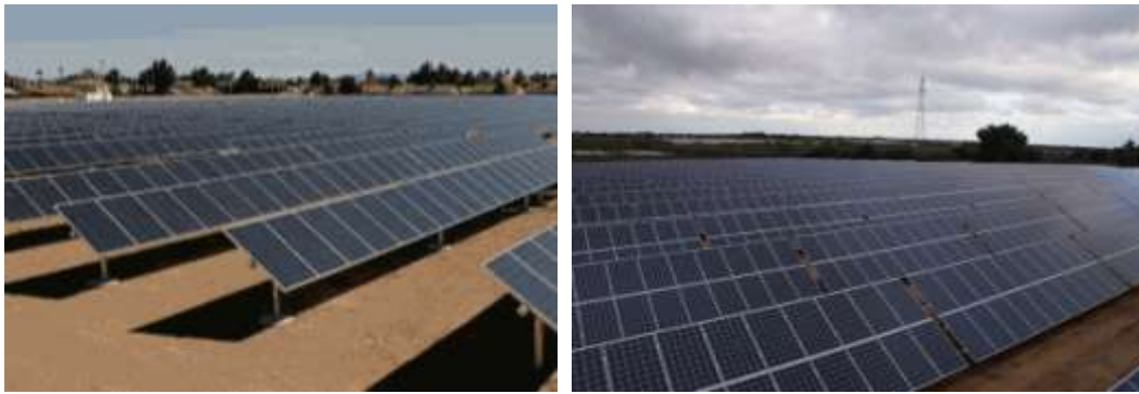
Figure 25: Showing typical positioning of solar arrays in a photovoltaic power generation facility (Solek, 2013).
