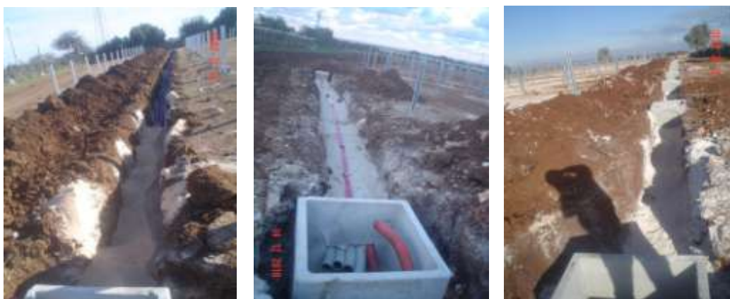
Figure 29: Examples of typical cable trenching used to connect the PV panels to the on-site substation (Solek, 2013)
