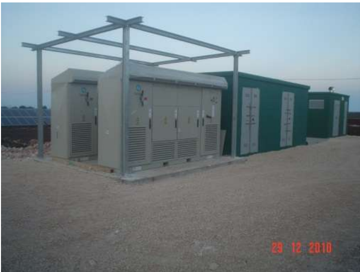
Figure 33: Showing typical example of on-site substation.
