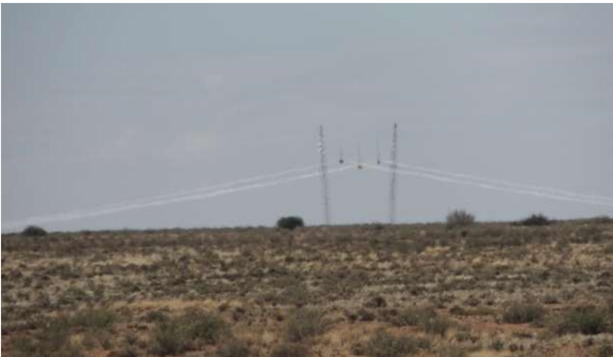
Figure 34: Photograph looking south of Eskom power line corridor that links to the Nieuwehoop substation.
