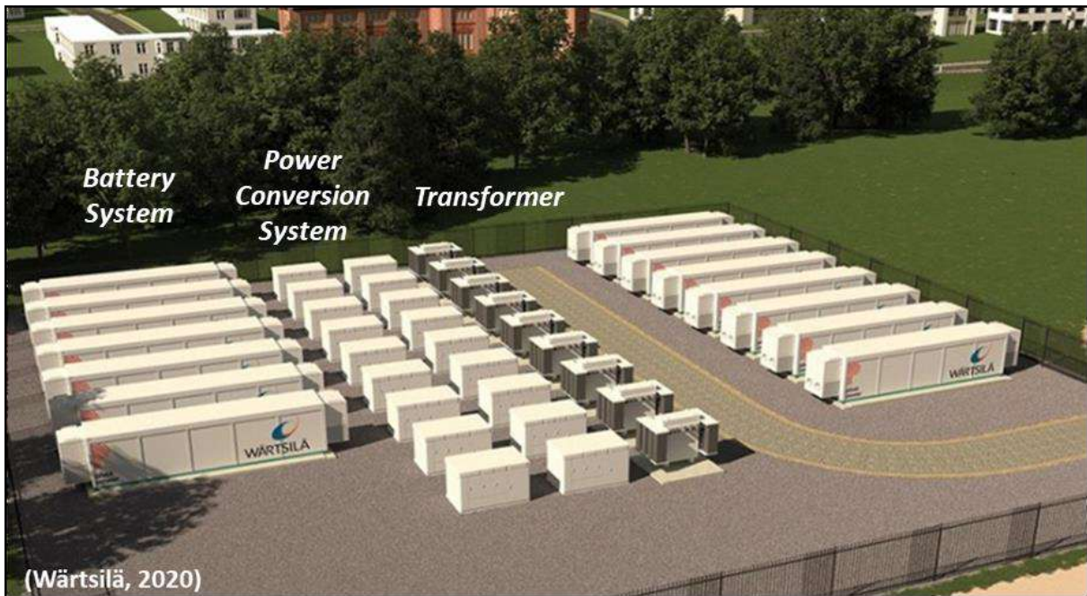
Figure 5: Example of a typical Battery Energy Storage System - Pivot Power's proposed lithium-ion battery in Kemsley, Kent.
