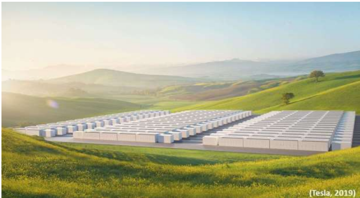
Figure 1: Tesla's Megapack Li-ion Battery (Modular System).
