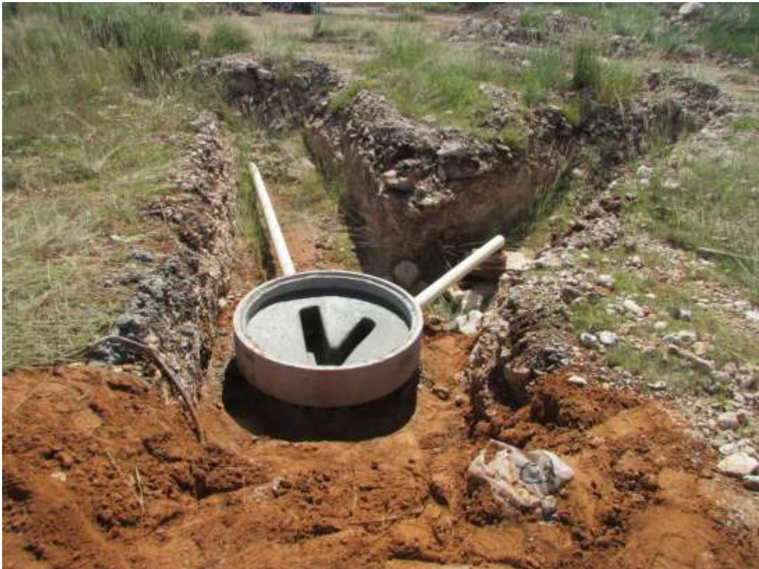
Figure 7: The installation of services is ongoing and being completed in some sections.
