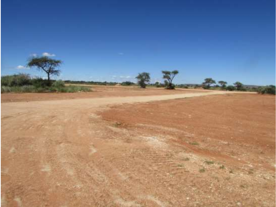
Figure 12: In some sections the installation of services and establishment of internal roads are completed.
