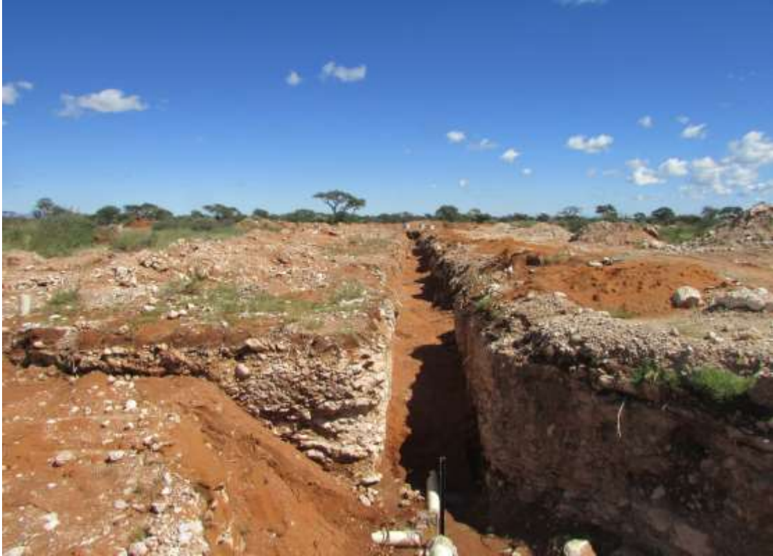
Figure 8: A view of one of the numerous open trenches in the area. Note the red sands and calcrete layers beneath.
