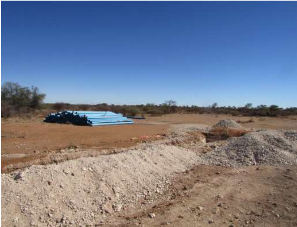
Figure 10: Another view of a section of the road showing trenches and pipe sections ready for laying.
