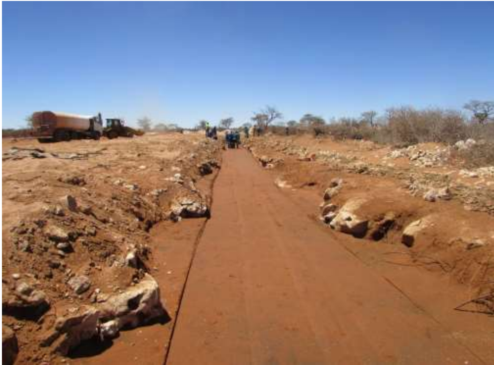
Figure 66: A view of a section of Trench 4. The trench is being filled again and compacted after the pipes have been laid.
