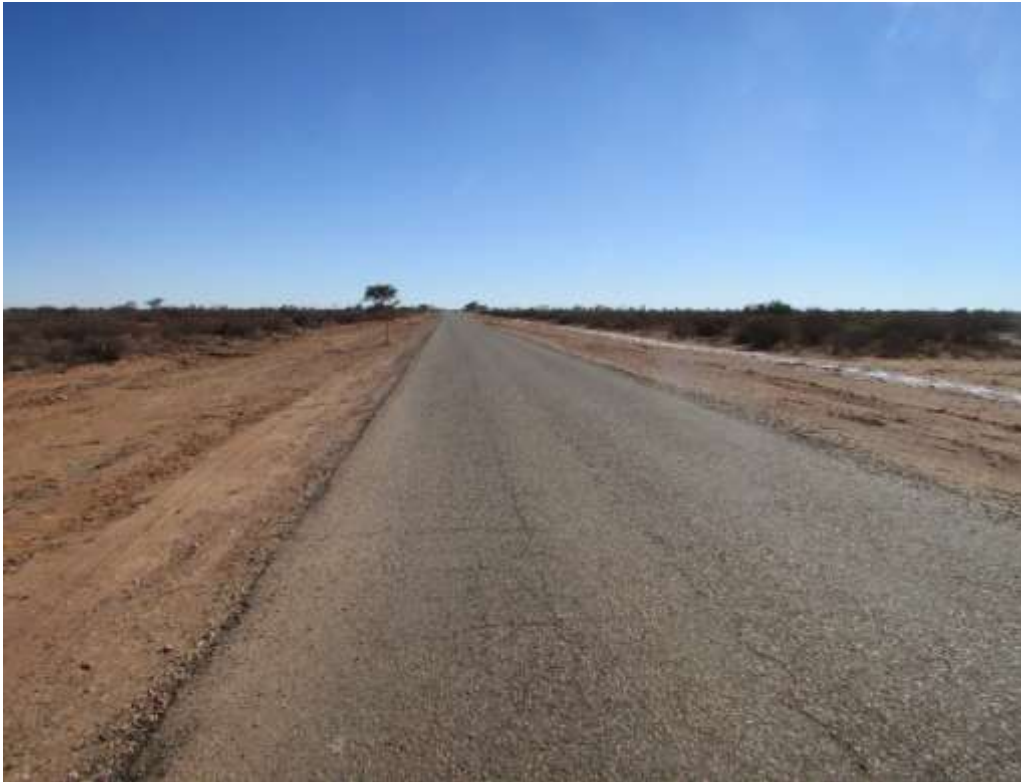
Figure 7: View of a section of the tar road in October 2019.
