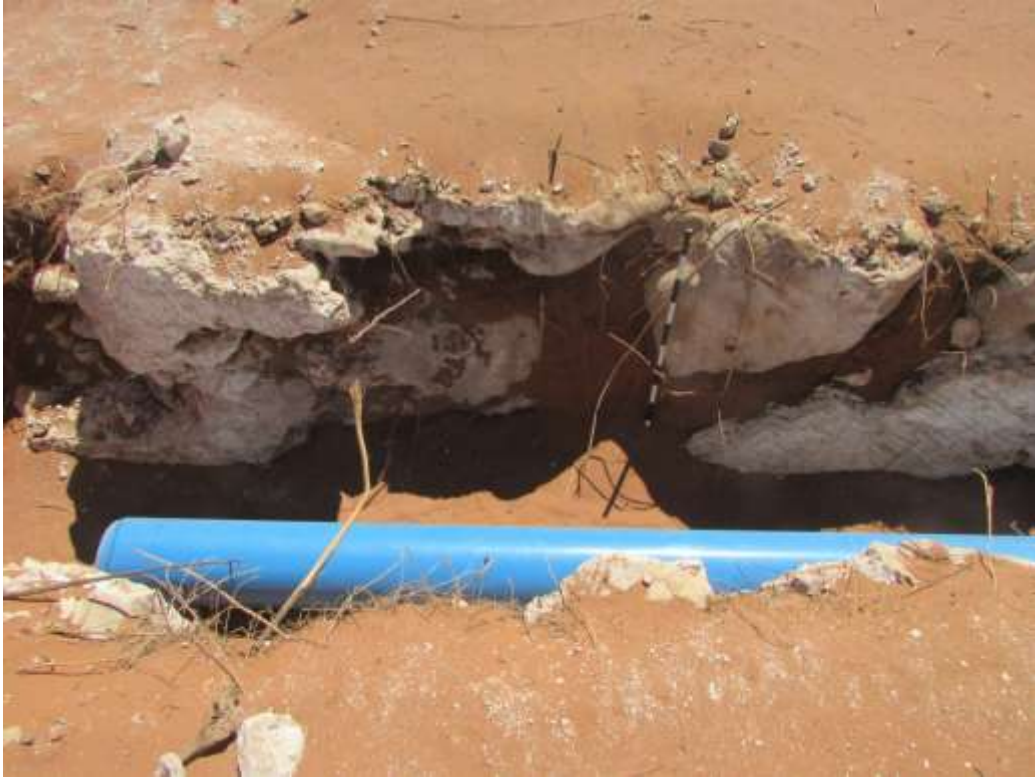
Figure 54: A section of Trench 1 with pipe showing red sand layer overlying calcrete formation below.
