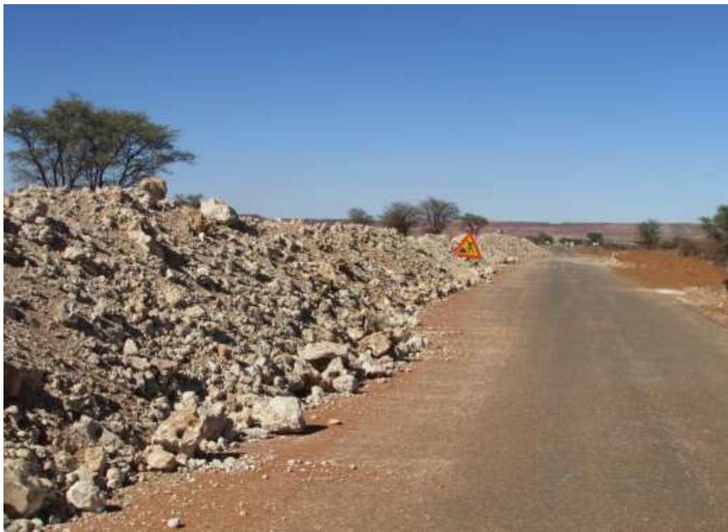
Figure 9: Another section of the road showing spoil heaps from trenches dug next to the road for pipelines.
