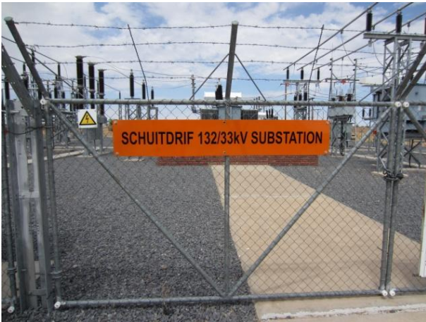
Figure 22: Existing Schuitdrift Substation
