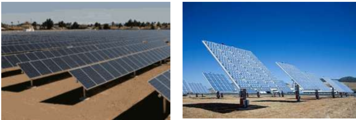
Plate 2: Showing typical examples of PV arrays (left) and CPV modules (right) (Solek, 2014)
