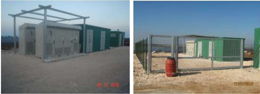
Plate 6: Typical example of on-site substation (Solek, 2014)
