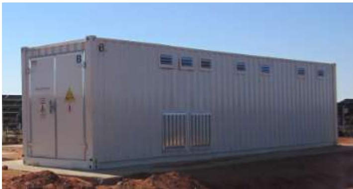
Plate 5: Typical example of inverter room (Solek, 2014)
