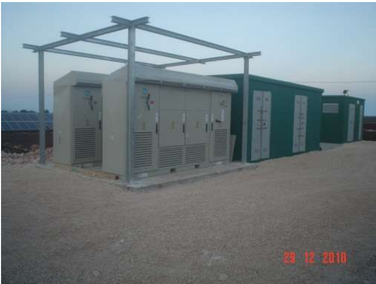
Plate 10: Typical example of on-site substation (Solek, 2014)
