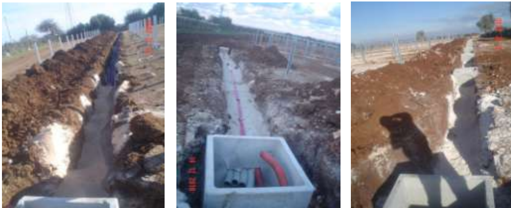
Plate 7: Typical example of internal cable trenching (Solek, 2014)
