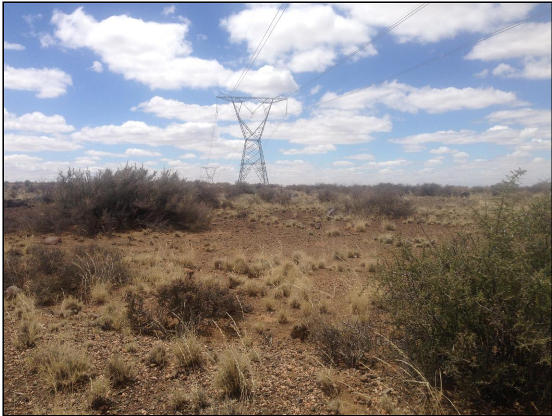
Figure 8: Existing Aries/Helios 1 400kV overhead power line.
