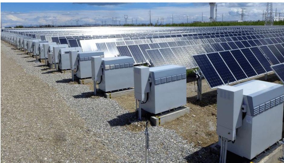
Figure 2.6: Example of battery storage units integrated as part of PV array (Source: nexttracker.com)
