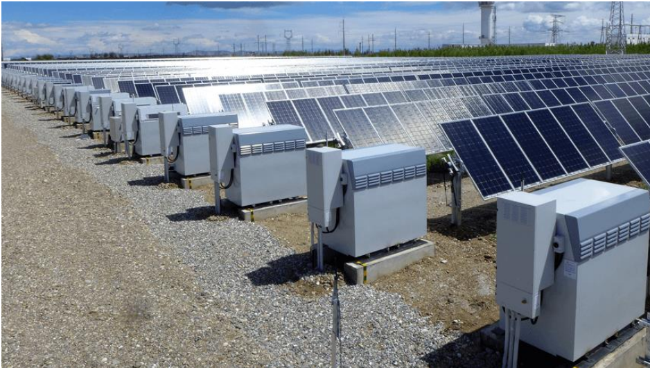
Figure 8.8 Example of battery storage units integrated as part of PV array (Source: nexttracker.com)
