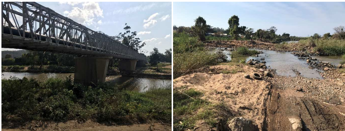
Figure 3-47: Existing iLovu River steel bridge (left) with disturbed river banks and riparian vegetation (right)
