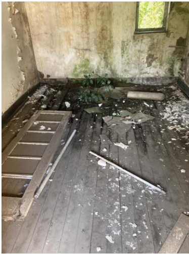
Photo 3 : Showing severe moisture damage to suspended timber floors.
