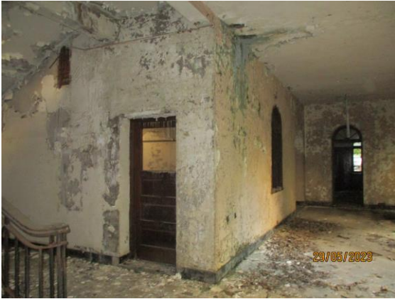
Photo 1 : Showing internal moisture damage.
