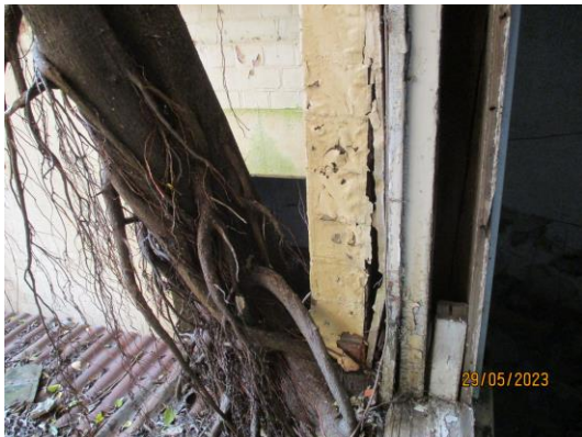
Photo 7 : Showing major vegetation growth affecting brickwork.
