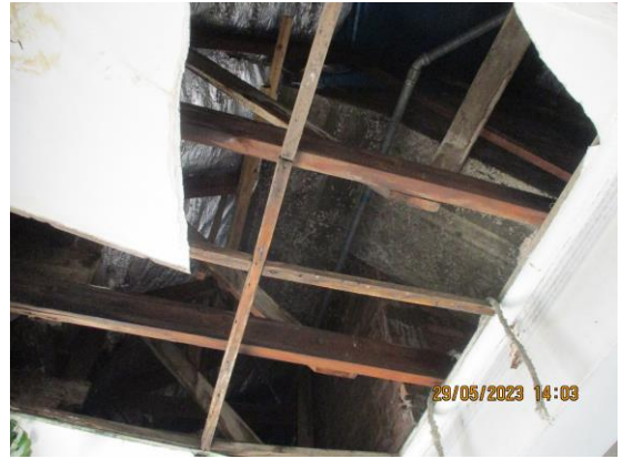
Photo 2 : Showing moisture damage to timber roof trusses and ceilings.
