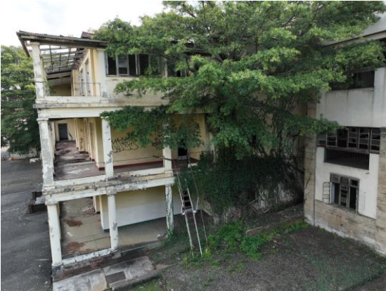
Photo 5 : Showing major external vegetation growth.
