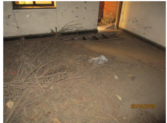
Photo 4 : Showing internal vegetation growth.
