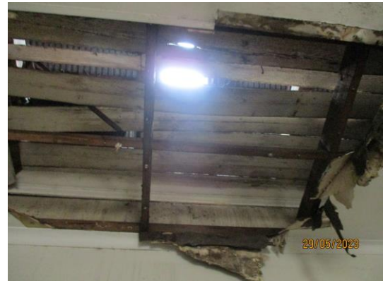
Photo 8 : Showing damage to suspended timber floors as well as roof covering.
