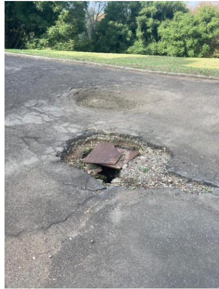
Photo 10 : Showing extensive damage to asphalt + subbase material around existing manhole.
