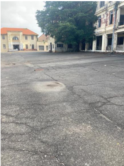
Photo 11 : Showing deterioration and 'crocodile cracking' to asphalt surfacing.
