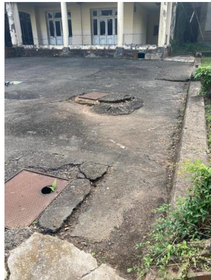
Photo 12 : showing heave + settlement between manholes.
