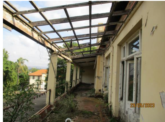
Photo 6 : Showing severely damage timber roof structure.
