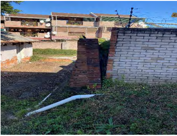
Photograph 21 : Showing the existing masonry boundary wall leaning / rotating.
