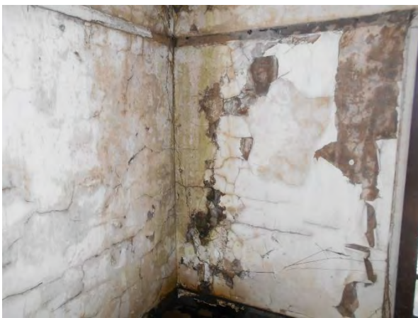
Photograph 5 : Showing severe moisture damage and cracks to the existing internal walls.
