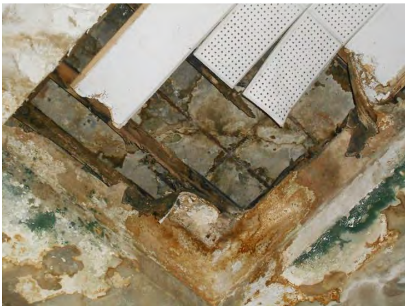
Photograph 17 : Showing severe spalling to the existing suspended concrete slab.
