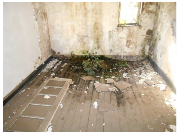
Photograph 6 : Showing severe moisture damage to the existing internal timber floors.
