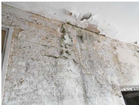
Photograph 7 : Showing severe moisture damage at the existing concrete slab and masonry wall interface.
