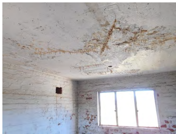
Photograph 8 : Showing severe 'leaching' of the existing concrete suspended slab in the mechanical lift shaft room.
