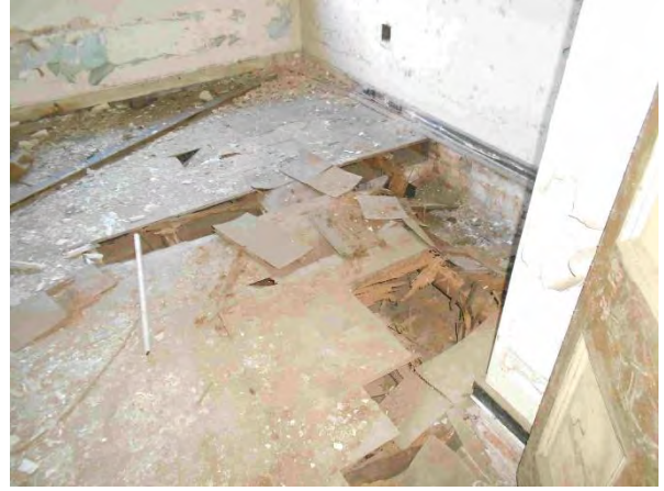
Photograph 2 : Showing severe damage to existing suspended timber floors.
