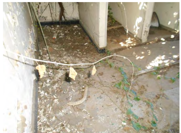
Photograph 18 : Showing severe settlement of the existing surface bed slab in the ablutions.
