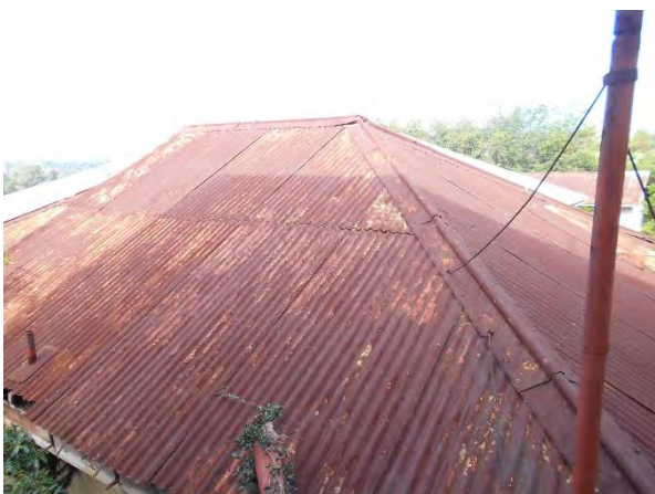
Photograph 11 : Showing the existing deteriorated and corroded metal roof
