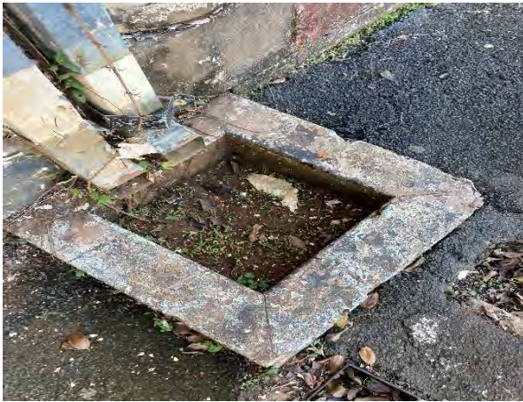
Photograph 23 : Showing existing silted stormwater gully.
