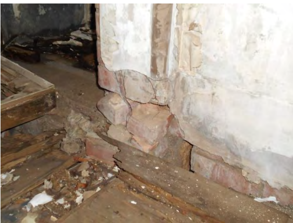
Photograph 3 : Showing damaged and loose brickwork below existing concrete column at first floor level.
