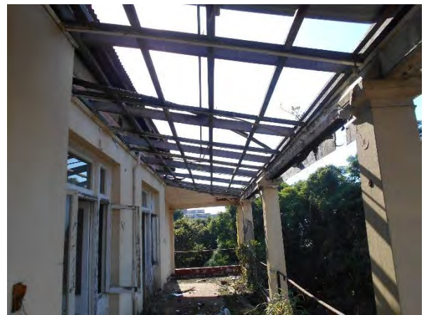
Photograph 10 : Showing severe damage to the existing timber balcony roof structure.
