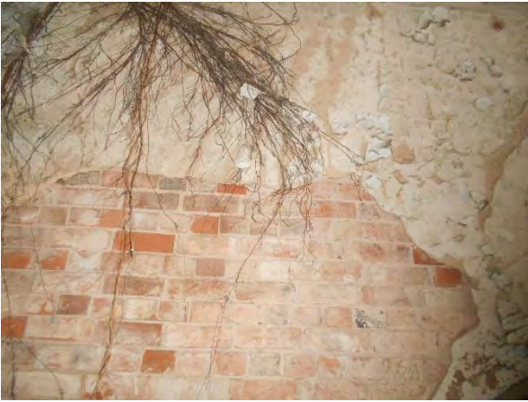
Photograph 1 : Showing severe delamination of plaster to internal walls.
