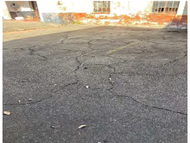
Photograph 24 : Showing severe 'crocodile cracking' of the existing premix layer.
