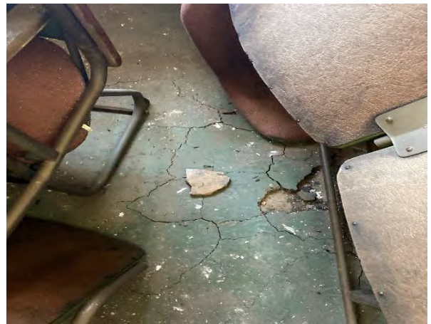
Photograph 14 : Showing severe damage to the existing screed on the suspended concrete slab.
