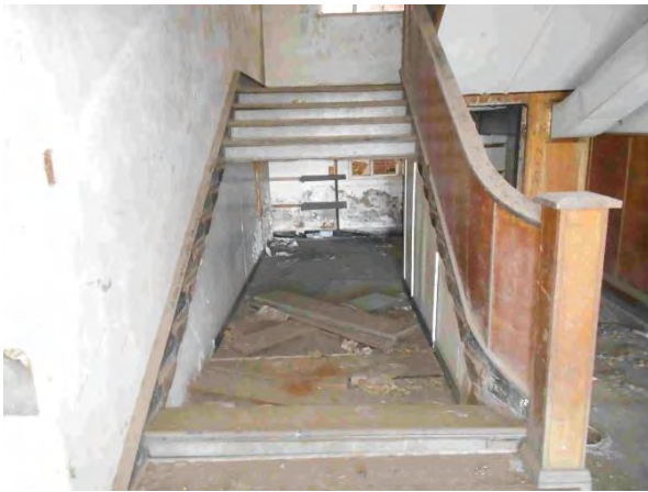
Photograph 9 : Showing the collapsed treads of the internal timber staircase.
