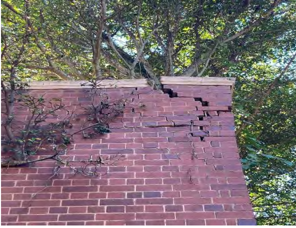
Photograph 19 : Showing severe structural damage to the existing parapet wall.
