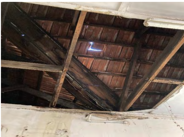
Photograph 13 : Showing damaged and displaced roof tiles as well as moisture damaged timber roof elements.
