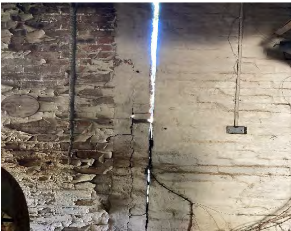
Photograph 15 : Showing separation of walls at the construction joint.
