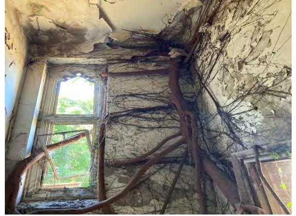
Photograph 20 : Showing severe vegetation growth internal of the building.
