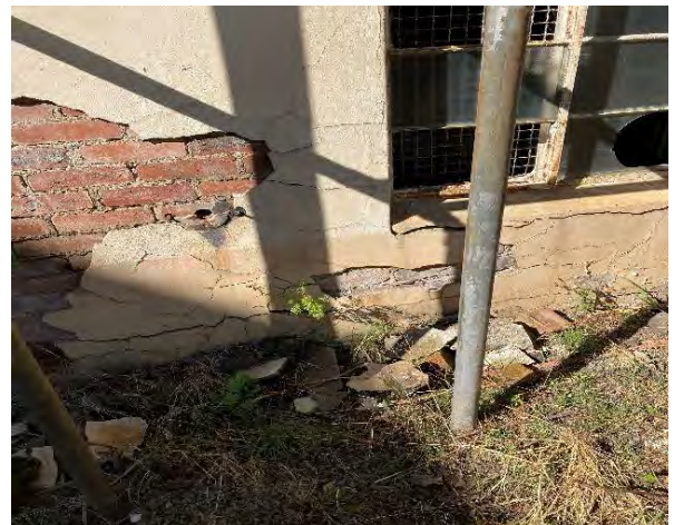
Photograph 16 : Showing delamination of the existing external plaster.
