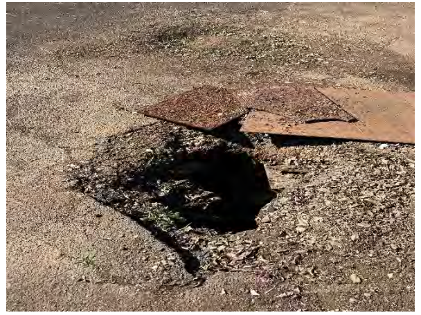
Photograph 22 : Showing severe damage to the premix and sub base layers around existing manholes.
