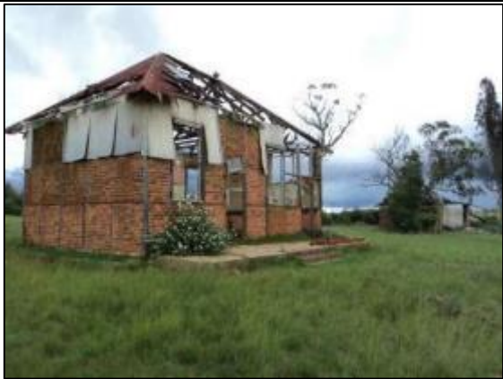
K12 – Dilapidated building.
