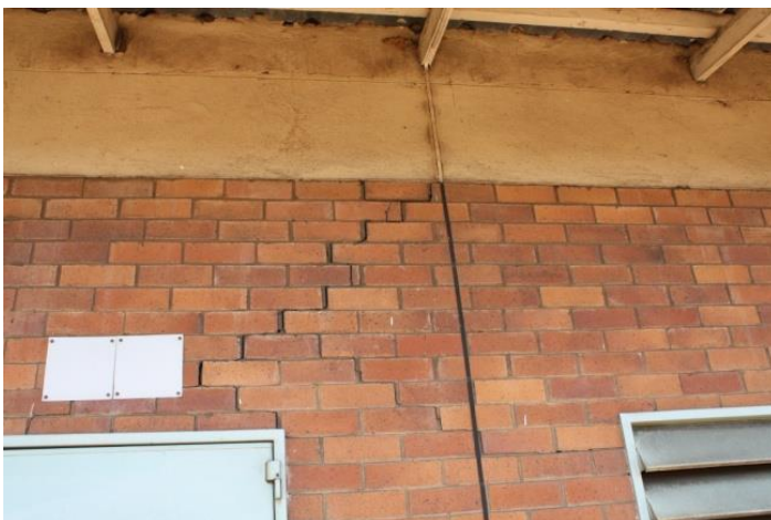
Figure 105: Example of blast induced damage.
