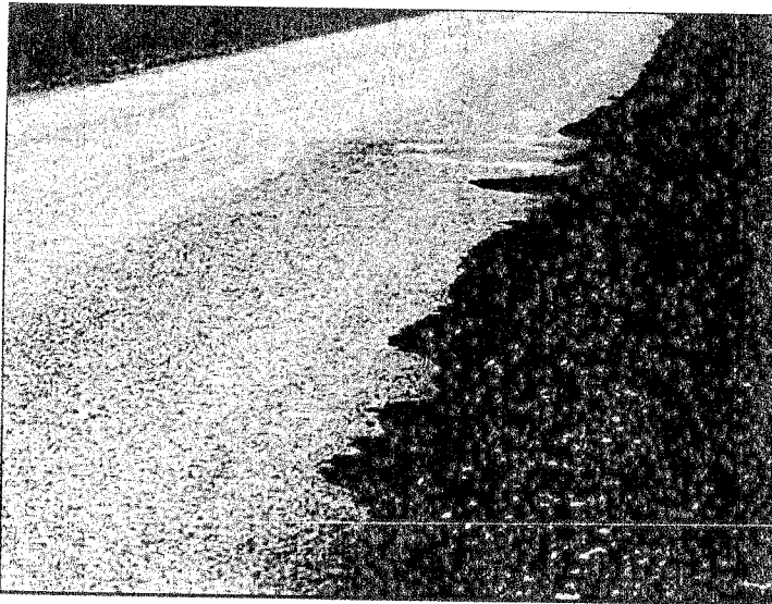
Figure 3-31: Major edge breaking on road surface
