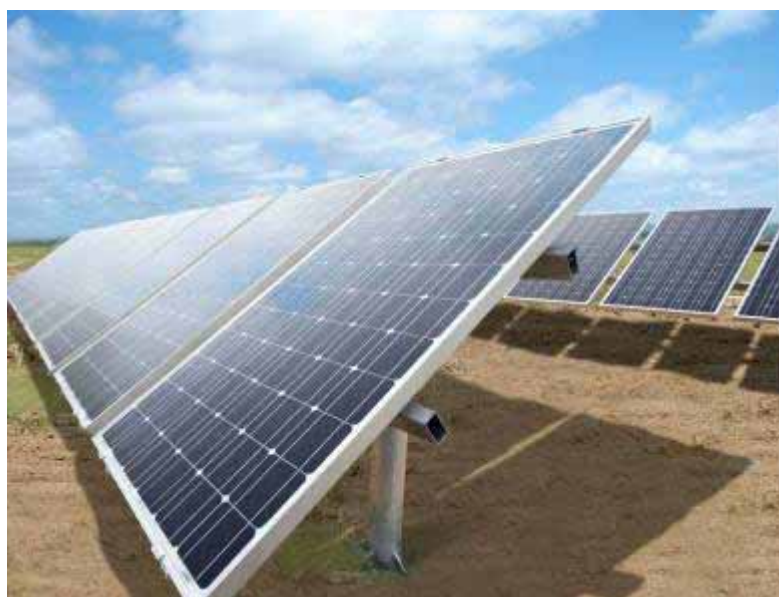
Figure 2.6: Photograph illustrating an array of PV panels.
