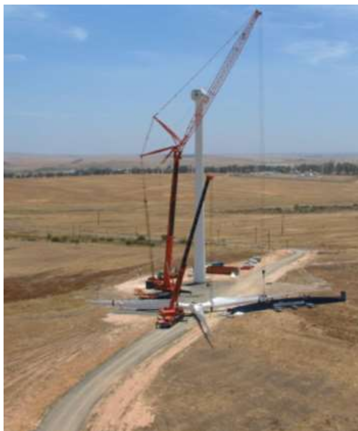
Figure 4.3: Photograph illustrating laydown areas required during the erection of one of the turbines at the Klipheuwel demonstration facility (photo courtesy of Eskom)
