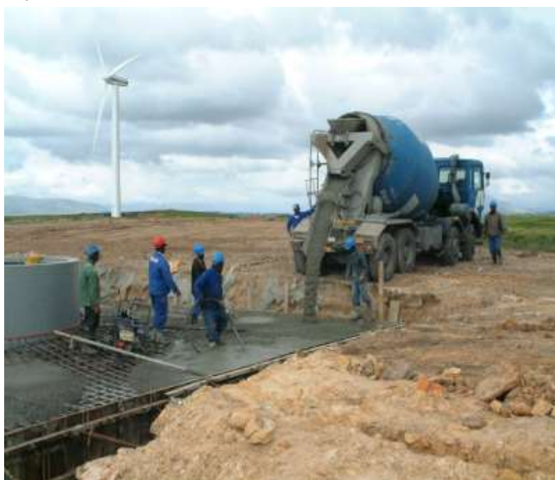
Figure 4.4: Photograph illustrating the construction of the foundation of one of the turbines at the Klipheuwel demonstration facility (photo courtesy of Eskom)
