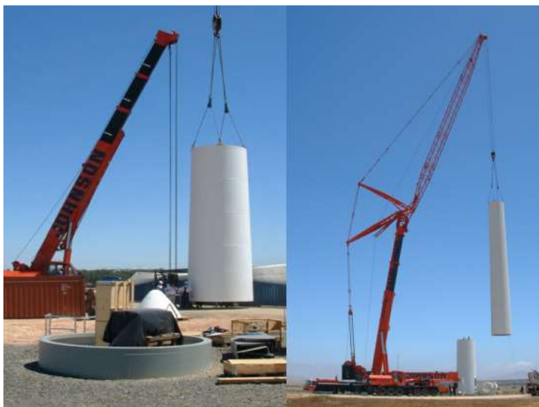
Figure 4.7: Photograph illustrating the assembly of a turbine tower utilising a large lifting crane (photographs courtesy of Eskom taken during the construction of the Klipheuwel demonstration facility)
