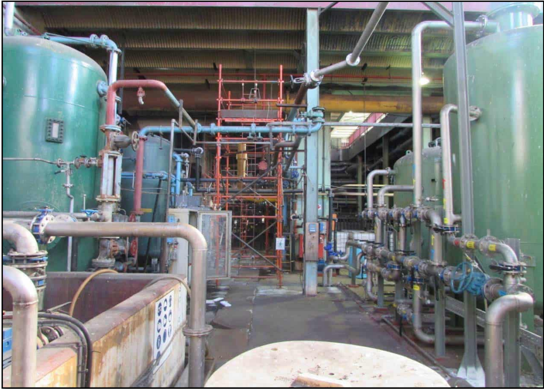
Figure 5: A view of a section of the inside of A-Station.
