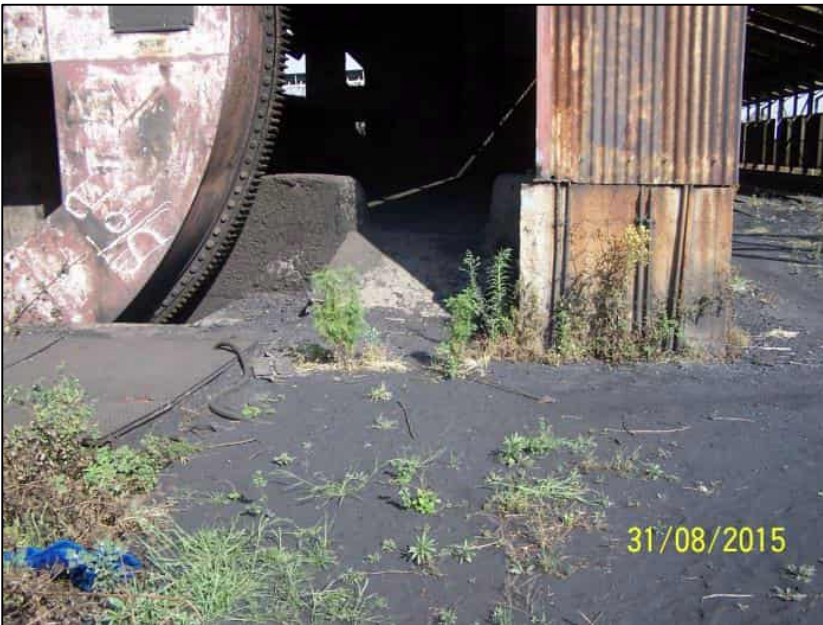
Figure 37: Coal residue on surface at Dry Coal Store
