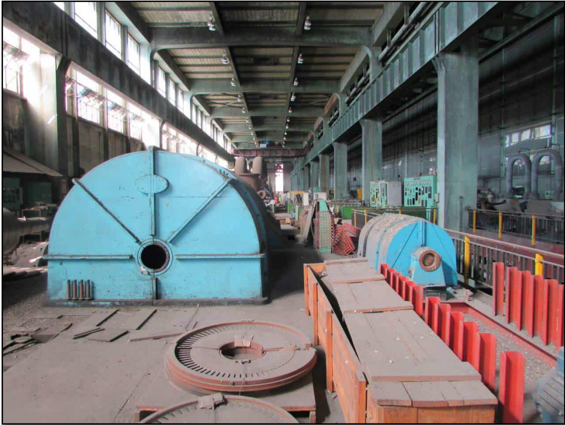
Figure 10: Another interior view of a section of A-Station and the machinery & equipmentt in it.
