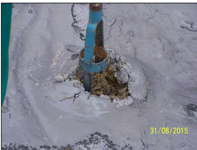
Figure 21: Auger sample at damaged concrete at Baghouse
