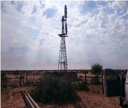
BH3 – wind pump
