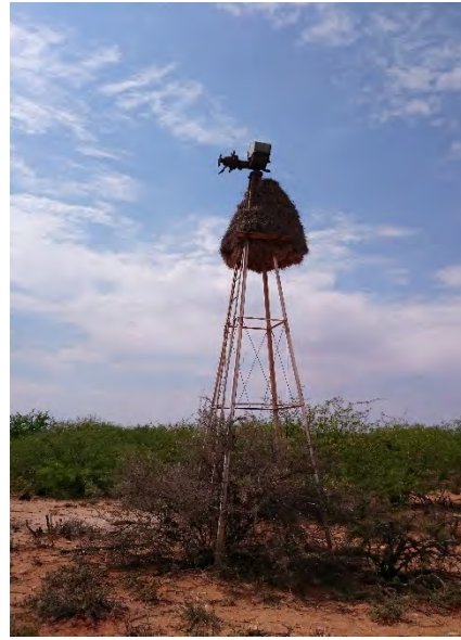
BH8 – wind pump
