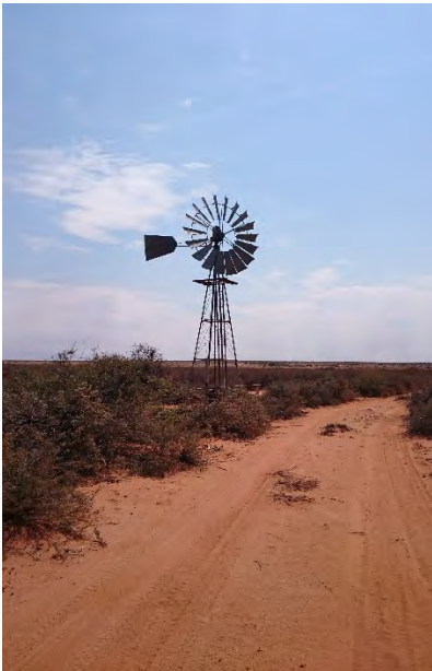
BH9 – wind pump
