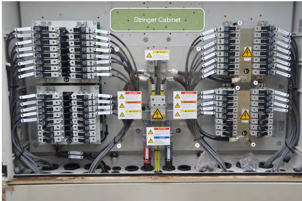
Figure 2: String Cabinet layout where supply from each panel is monitored.
