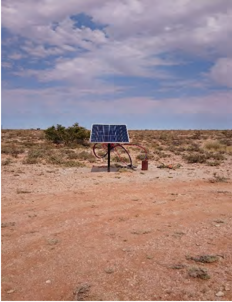
BH7 – solar pump borehole
