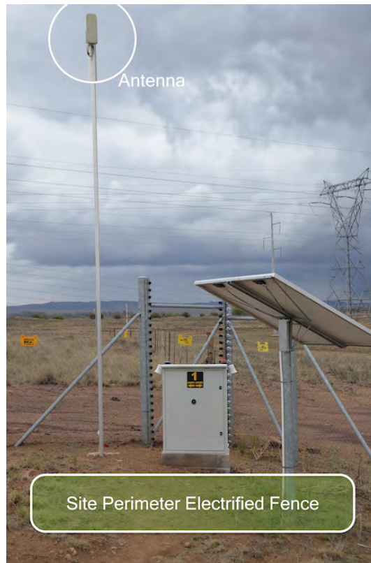
Figure 36: Electric fence surrounding the perimeter of the Dreunberg PV plant.
