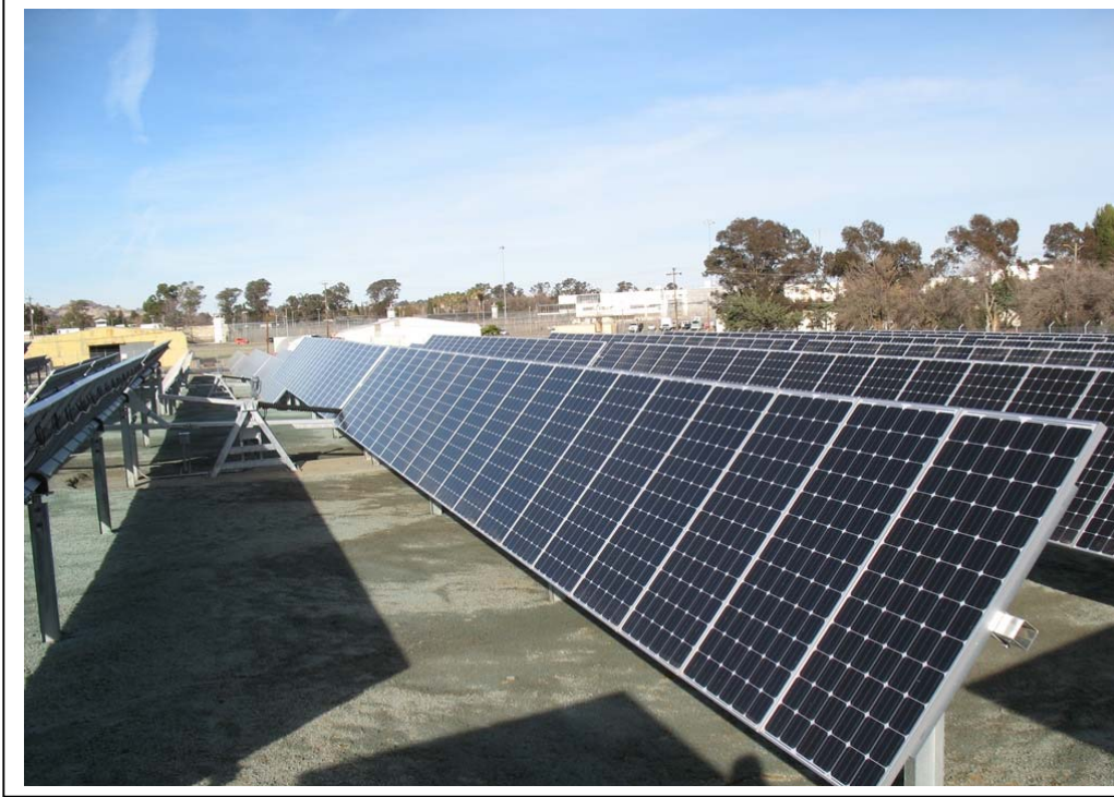
Figure 2.6: The support structures elevate the PV panels and allow for single axis tracking of the sun for increased efficiency (Source: Gestamp Asetym Solar South Africa (Pty) Ltd)
