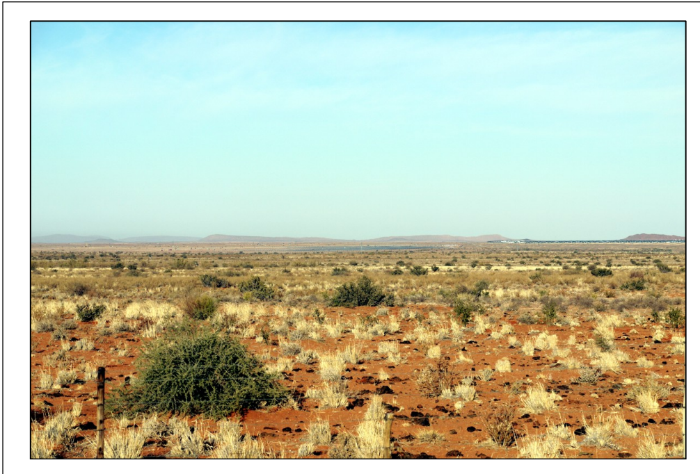
Figure 7.20: View of Sirius Solar PV One project under construction (centre picture) from the Lutzputs Road.
