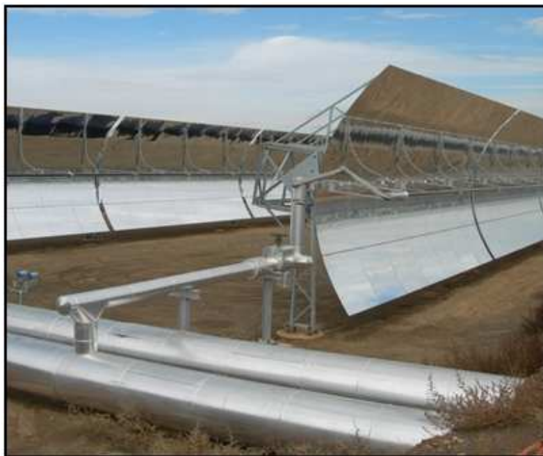
Figure 1: Parabolic trough solar collector assembly
