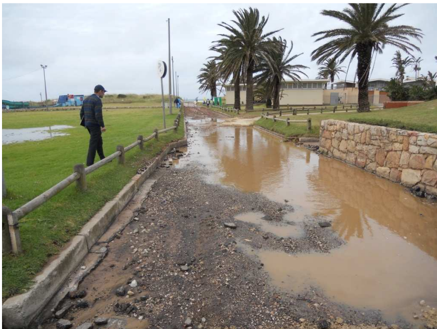
Figure 2: A view of the current access path to the beach that runs south of the Supertubes after heavy rainfall.
