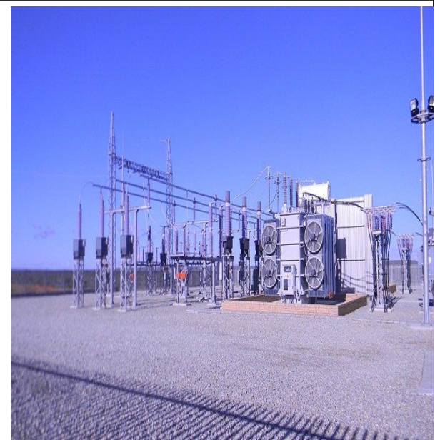
Photograph 7.4: Substation (Sere Wind Facility)
