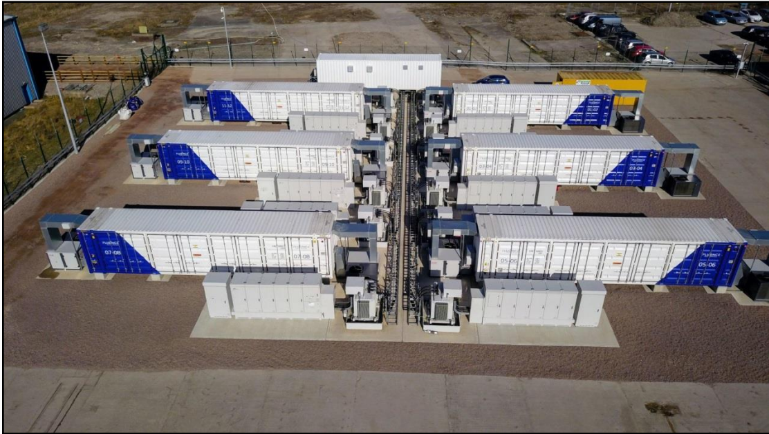
Figure 3: Aerial view of a BESS facility (Photo: Power Engineering International).
