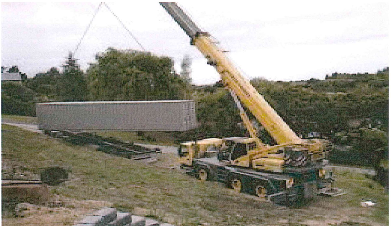
Photo 6: Typical handling and off-loading of Shipping Containers on Site, using Mobile Cranes
