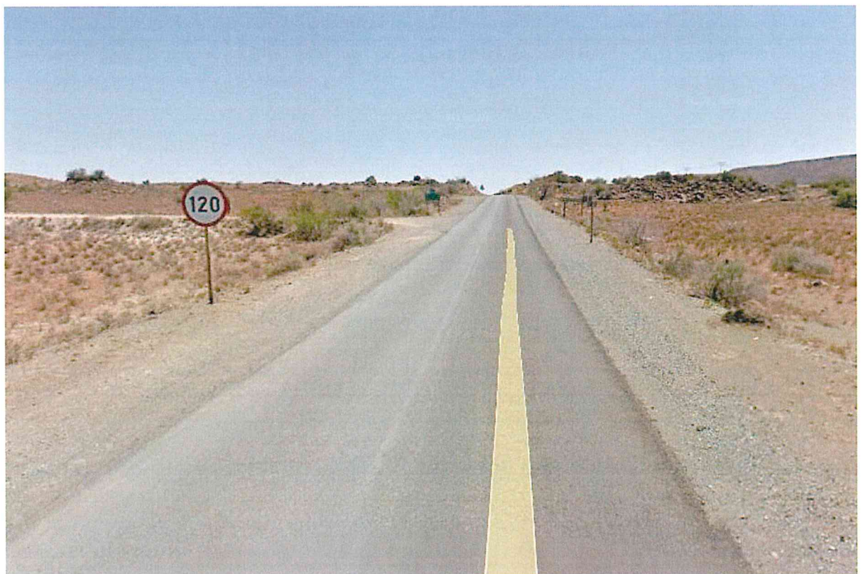
Photo 10: : Northern view Provincial Main Road (R48) north of Petrusville. Note that no surfaced shoulders exist (only gravel shoulders) and no or poor line markings exist.
