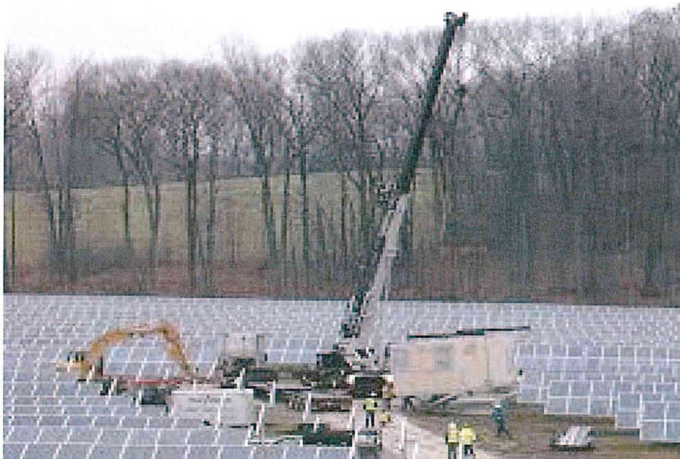
Photo 7: Typical handling of Shipping Containers and PV Solar Panels at point of installation. Note the space required for mobile cranes to manoeuvre during the installation process.
