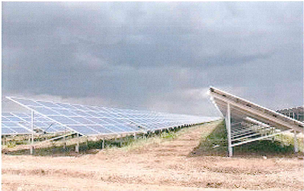
Photo 20: View of typical Internal Service Roads in-between arrays of PV Solar panels. Note the condition of good rehabilitated roads.
