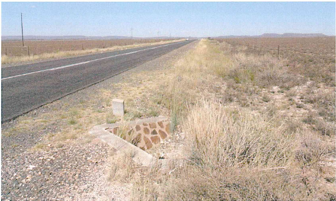
Photo 13: Easterly view of Provincial Main Road (R369) at the position of 'Site Access No.2'. The northern parts of Farm RE/18 is situated on the right (south) of this provincial road. Note the storm water inlet structure, collecting over-land flow from the proposed development areas.
