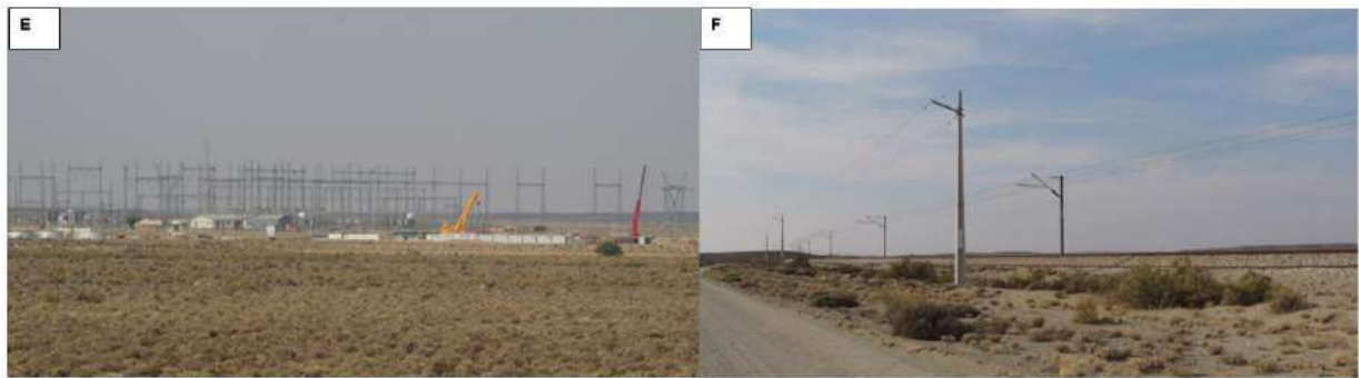
Figure 6-25:| E: Photograph of the Eskom Helios Substation; F: Photograph of the overhead electrical structures and cabling associated with the Sishen-Saldanha railway line.
