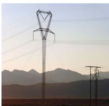
Plate 2-5: Guy line supported steel structures.
