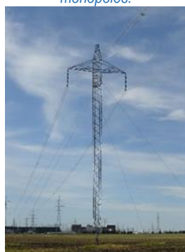
Plate 2-6: Free standing metal lattice towers.
