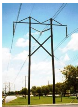
Plate 2-7: Multi-pole structures such as H-towers or K-towers.
