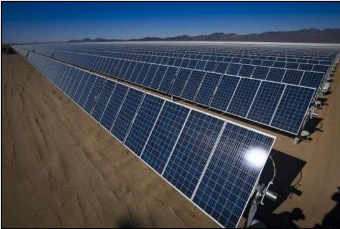
Photograph 1.1: Typical PV SEF facility
