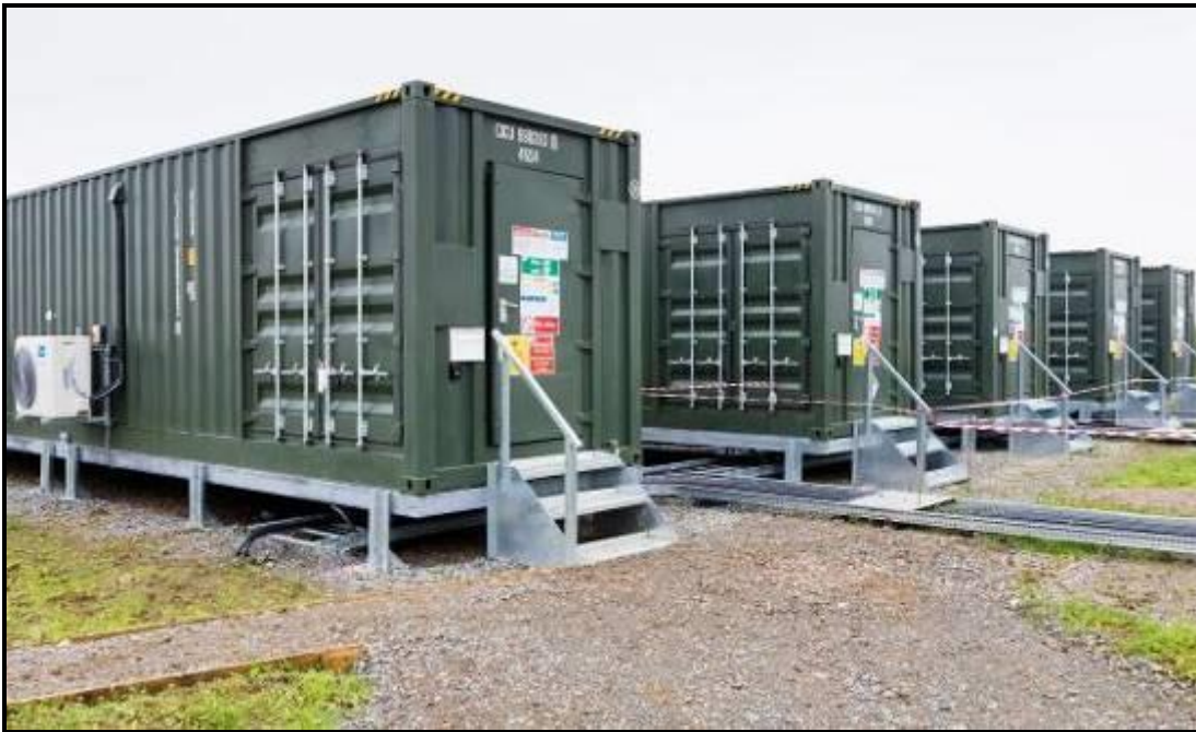
Photograph 1.2: Example of BESS located in storage containers
