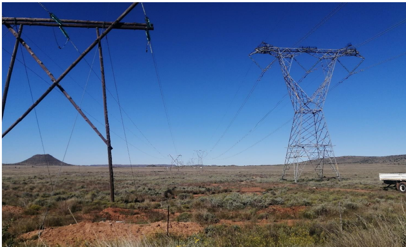
Figure 10: Electrical infrastructure that traverses the study area
