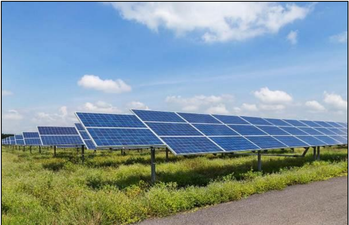
Photograph 1.1: Typical PV SEF facility
