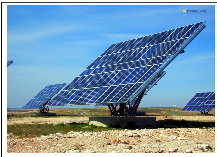
Figure 3.3: The support structures elevate the panels and allow for dual axis tracking of the sun for increased efficiency (Source: Gigaom)
