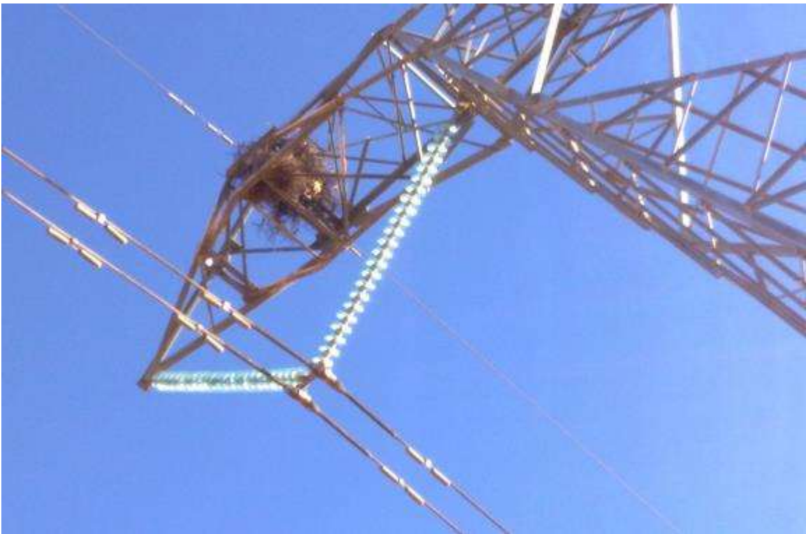
Figure 2: The inactive Martial Eagle nest at the site on tower 147 of the Aggeneys – Aries 400kV.
