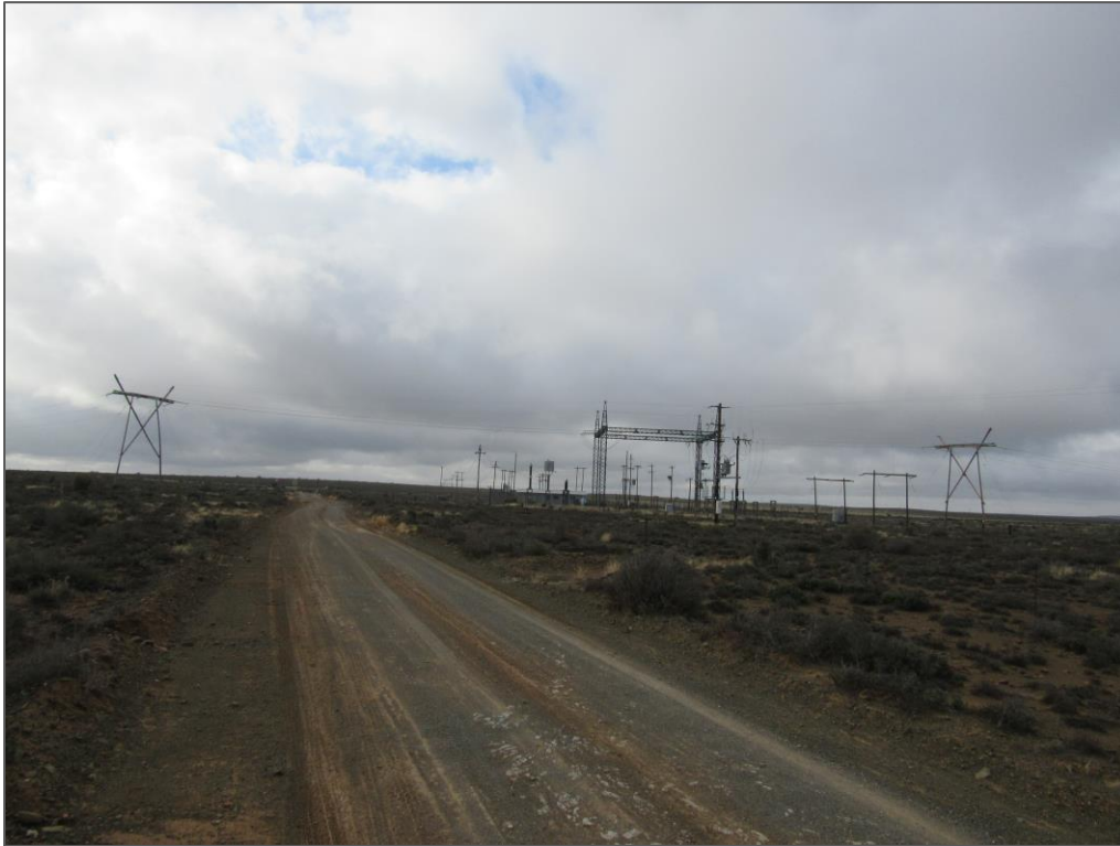
Figure 19: 22kV power lines and associated substation north of the Kraaltjies WEF application site, adjacent to the N12.
