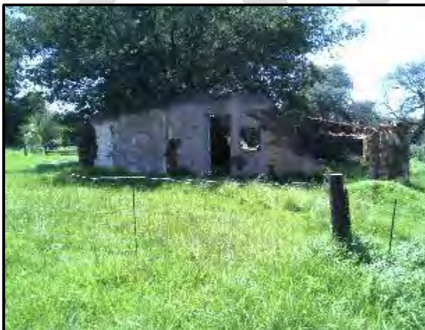
Figure 28. Dilapidated structure at KP 15.
