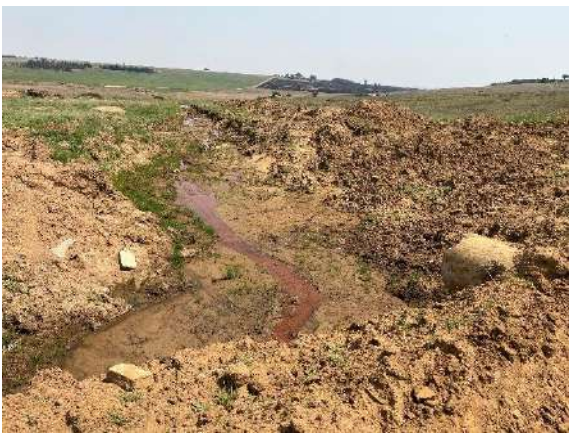
Excavations within a wetland just outside of the southern boundary for the MRA area to facilitate a road crossing.
