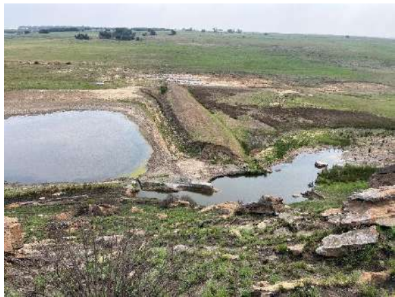
A seemingly purposefully beached impoundment wall that has impacted on the ecological integrity of the valley bottom wetland unit.
