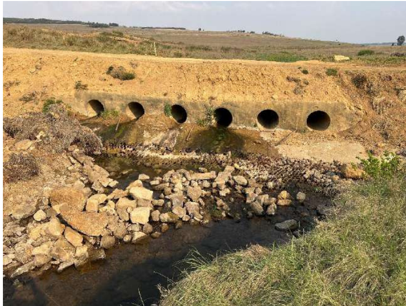
Figure 24: Poorly designed road crossings create migratory barriers to fish and impact fish populations through habitat fragmentation (the bridge crossing point associated with site 4).
