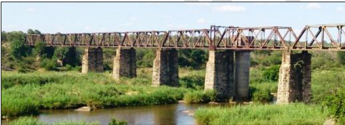
Figure 7: The Selati Railway Bridge with its sandstone pillars and the pump house (© K. Zunckel).
