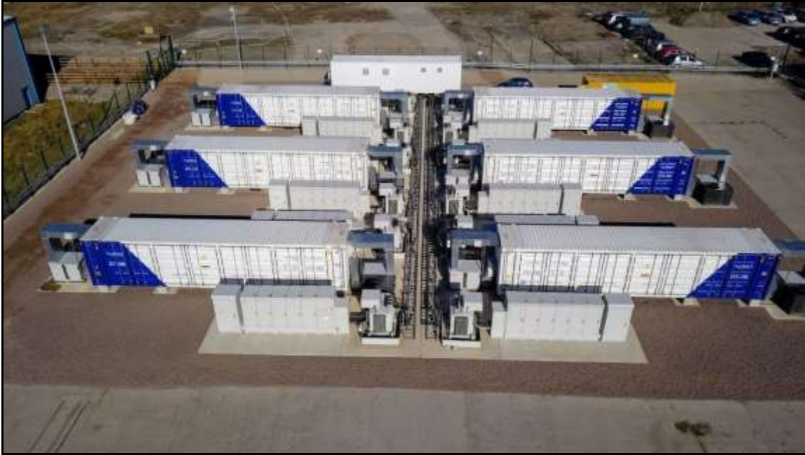
Photograph 1.2: Example of BESS located in storage containers
